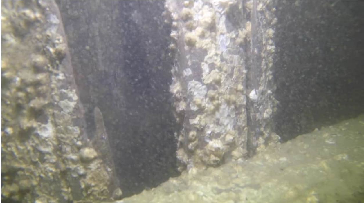
Pile 30E Severe Damage - timber pile hollow from surface down to base
