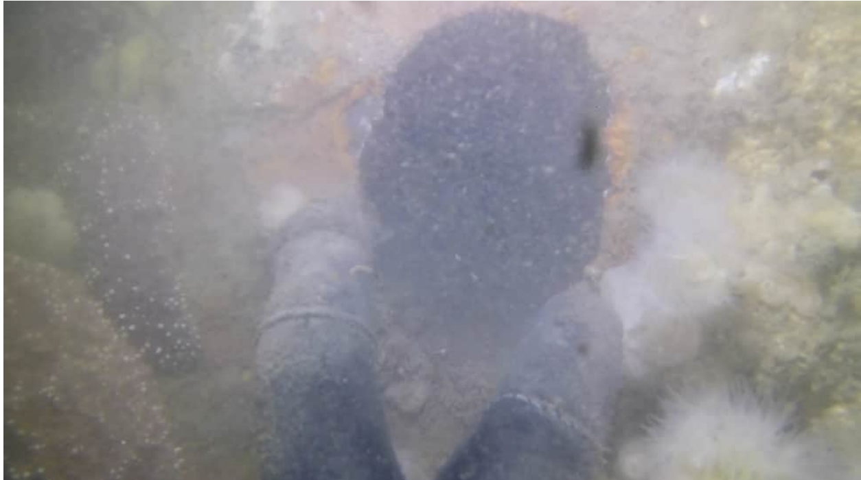
Pile #NC1 Moderate Damage - steel pile with hole
